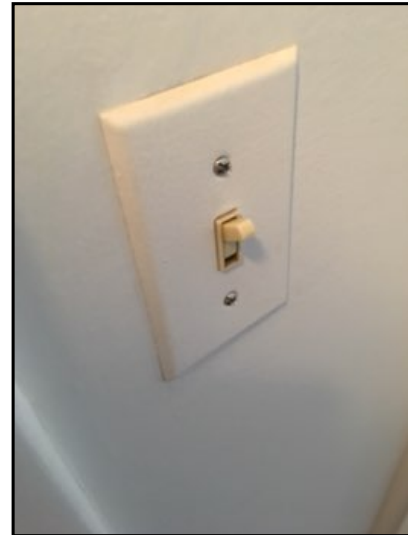
3 way switch not working properly
