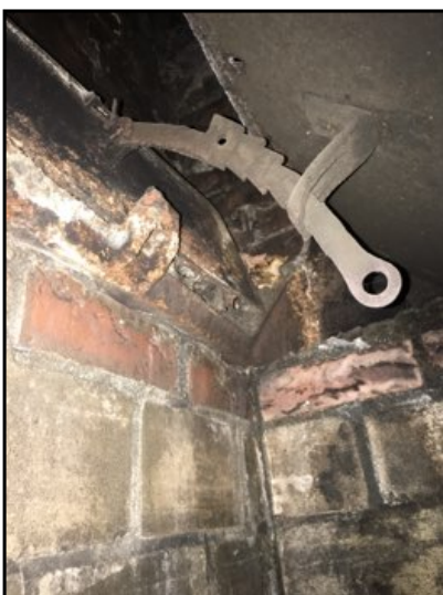
Leaves and debris in chimney
