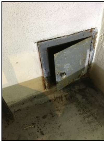
Clean out door will not stay closed
